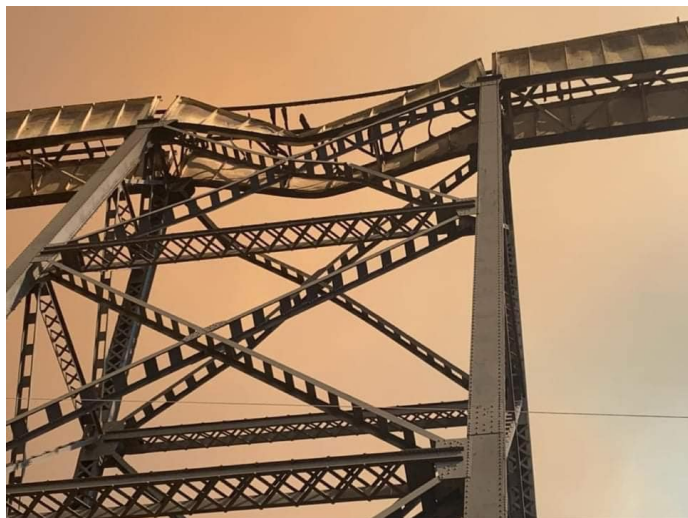
The Union Pacific Dry Creek Trestle with major post-fire structural damage, June 2021.
