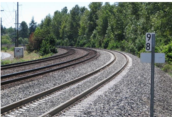
The new third main track is in place south of the Kelso station but is not in service yet, pending completion of other nearby construction. Three photos by Jim Hamre
