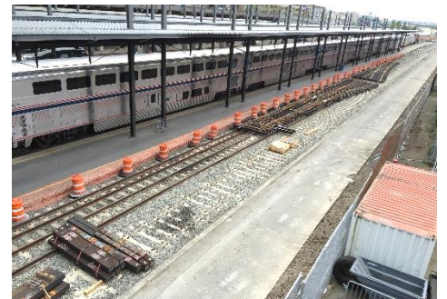
Construction of Track 7 and upgrading the south approach at King St. Station are underway. The 19th century hand thrown switches will finally become history in the 21st century.
