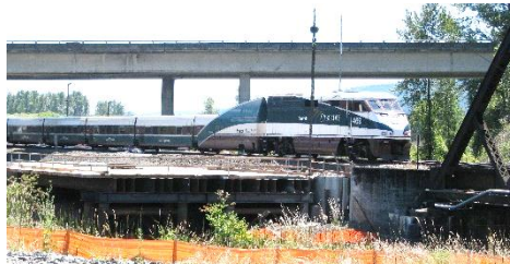
Cascades 506 crosses the Coweeman River, where a new bridge for the Kelso third main train is under construction.
