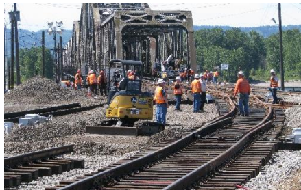
BNSF rebuilds the junction in Vancouver, WA in April 2015. Major track changes here will speed freight and passenger train movements.
