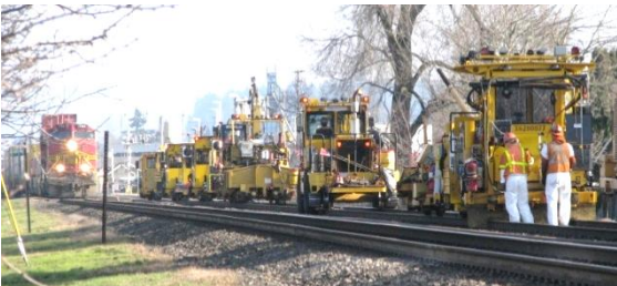
BNSF crews perform regular track maintenance in Puyallup in late January. WSDOT funds additional work to speed up the corridor improvements. Photo by Jim Hamre
