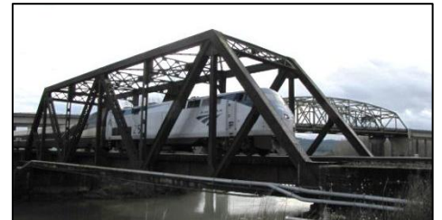
Amtrak Cascades train 516 crosses the Coweeman River near Longview Jct. in Feb. 2011. The Kelso to Martins Bluff project will build another bridge over the river as part of the construction of a third main track in this area.
